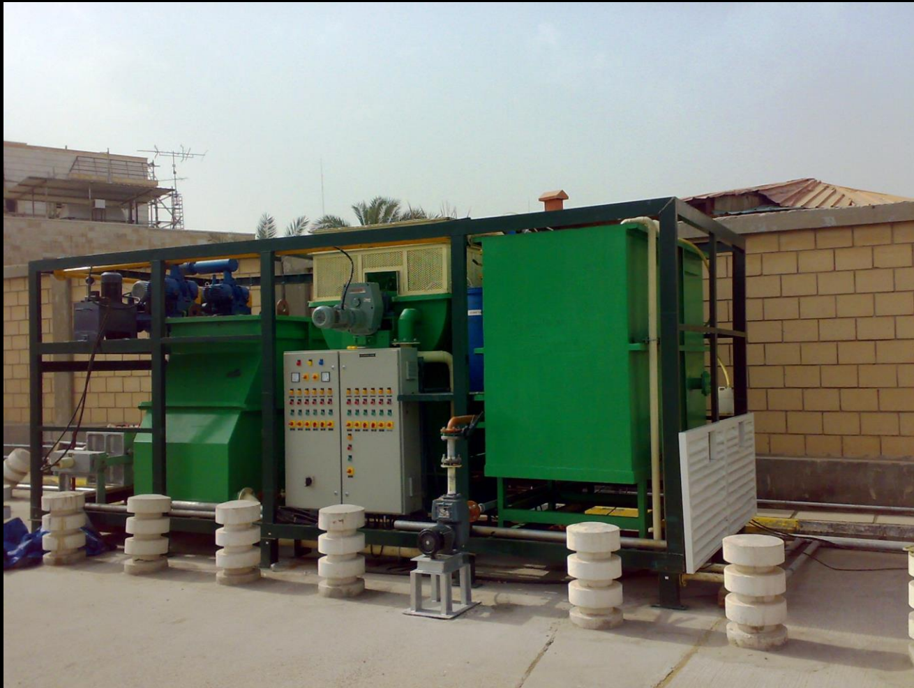
2008: 100cmd plant for Automobile service station at Bayan, Kuwait
